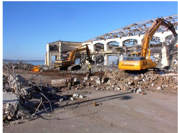
Stilwell Hall, Ft. Ord, CA. During demolition, there was only a narrow window of time to operate since the building was located in a sensitive habitat area.
