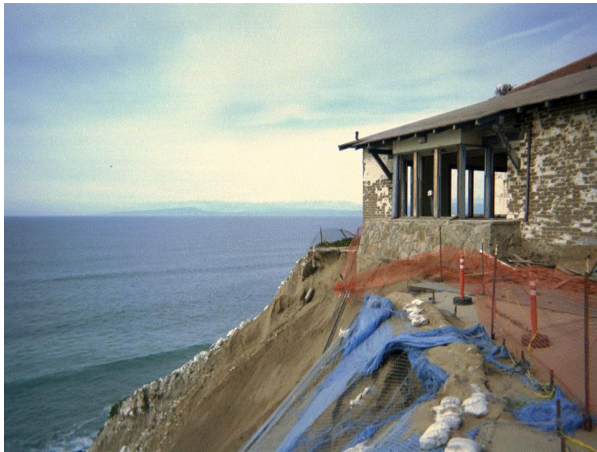
Stilwell Hall, Ft. Ord, CA. Due to years of heavy storm activity, the cliffs were badly eroded, undercutting the former Officer's Club building, which was threatening to fall into the bay.
