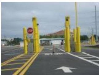
Port of Panama City, FL. Radiation portal monitor pair.
