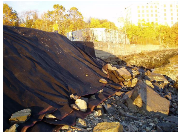
Portsmouth Naval Shipyard, Kittery, ME. Ahtna performed all construction activities, including removal and replacement of embankment and placement of zone material on slopes.
