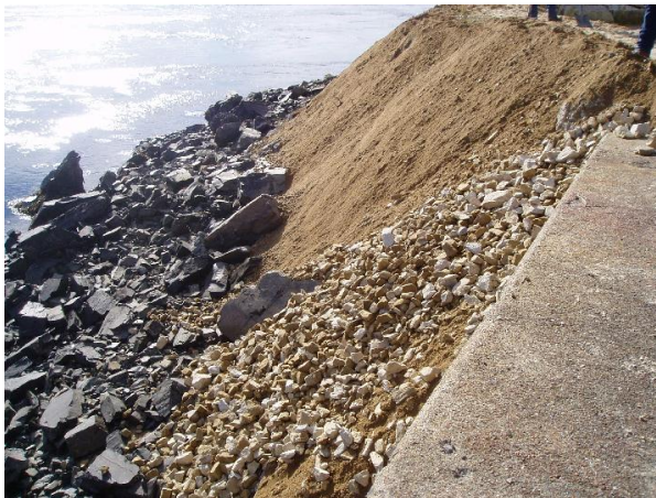
Portsmouth Naval Shipyard, Kittery, ME. Significant erosion was discovered along the shoreline at the facility adjacent to the DRMO Salvage Area.
