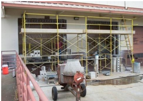
Commissary Dock Repair, Hickam AFB, HI. Ahtna's CMU wall repair in progress.
