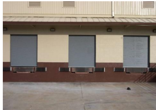
Commissary Dock Repair, Hickam AFB, HI. Ahtna's completed repairs included installation of new roll-up doors and new loading dock bumpers.
