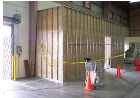
Commissary Dock Repair, Hickam AFB, HI. Ahtna constructed a false wall to protect products in the delivery area.
