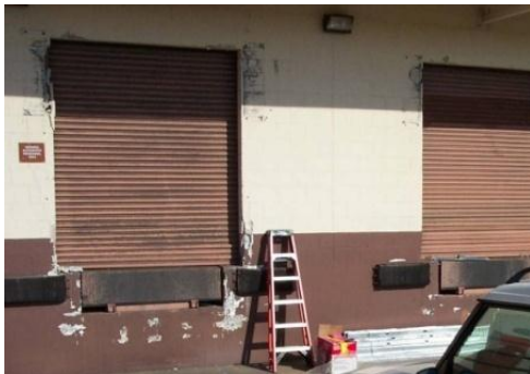
Commissary Dock Repair, Hickam AFB, HI. Damaged CMU walls and old roll-up doors prior to the start of Ahtna's repairs.
