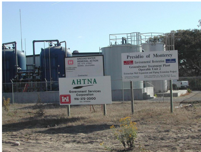
Groundwater Treatment System Operation and Maintenance, Former Ft. Ord, CA. The GWTPs consist of 38 extraction wells and six injection wells and infiltration galleries.
