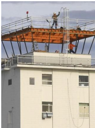
Billings Logan International Airport, Billings, MT. Air traffic control tower roof replacement.
