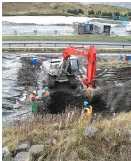
Chevron Site Remediation, Dutch Harbor, AK. Ahtna's excavation of the trench consisted of the removal of contaminated soils and screening and storage in the temporary cell.
