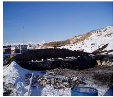
Chevron Site Remediation, Dutch Harbor, AK. This entire project was completed in the most severe weather conditions: snow, rain, and winds of 100 miles per hour.
