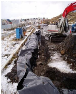
Chevron Site Remediation, Dutch Harbor, AK. Ahtna lined the trench with 20-mil liner to restrict and redirect water.
