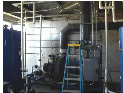
Groundwater Treatment System, Dinuba, CA. Interior view.
