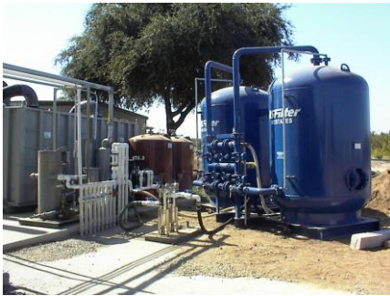
Groundwater Treatment System, Dinuba, CA. Ahtna provided system design; cleaning, removal, and disposal of the above ground tanks; and construction of the new system.
