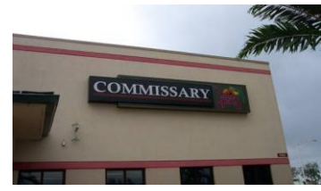
Schofield Barracks Commissary, Oahu, HI. Ahtna installed an internally illuminated commissary sign on the outside of the commissary.
