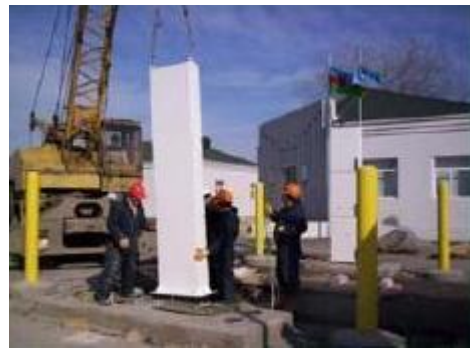
Shirvanovka, Azerbaijan. Radiation Portal Monitor placement.
