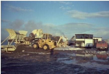
Cold Bay, AK. Ahtna provided excavation and thermal treatment of fuel-contaminated soil in Cold Bay. Cold Bay, known as the “Gateway to the Aleutians,” was the site of a former Air Force Tank Farm.
