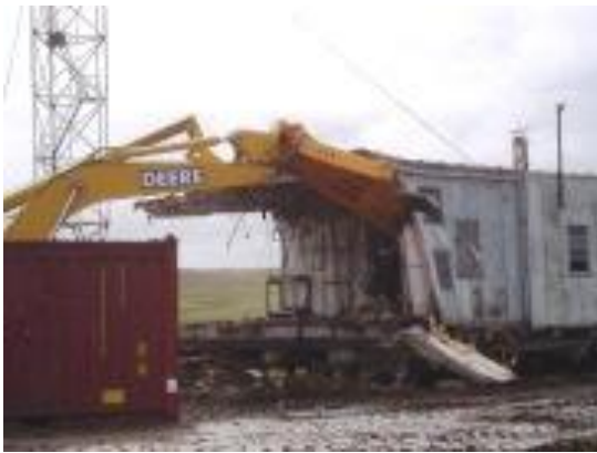
Cape Sabine, AK. Ahtna carefully performed demolition of buildings, tanks, and towers taking care not to damage the sensitive Alaskan tundra.
